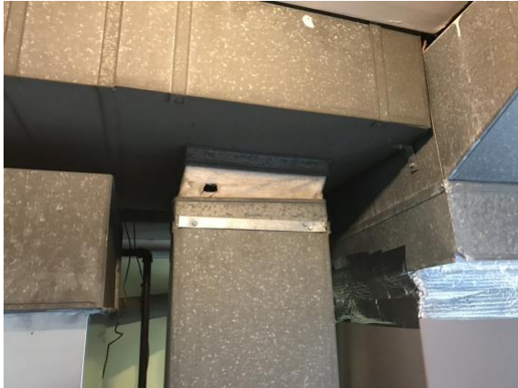
Fabric dampener on return duct
