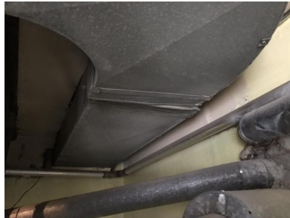
Fabric dampener on supply duct
